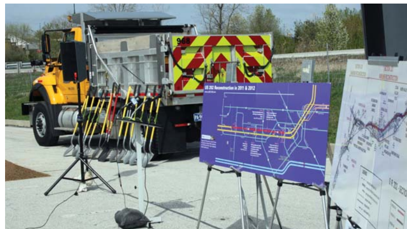
Construction has begun on US 202—Section 320 to widen and reconstruct from North Valley Road to Mill Lane.
